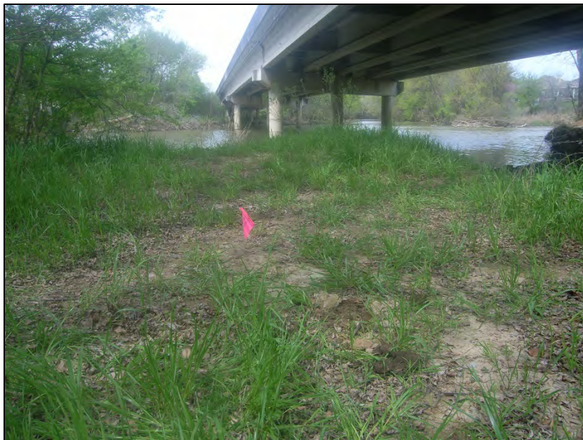
Photo ID 20: View of Crossing 1, Village Creek and associated wetland, located between westbound I-20 main lanes and frontage road.
