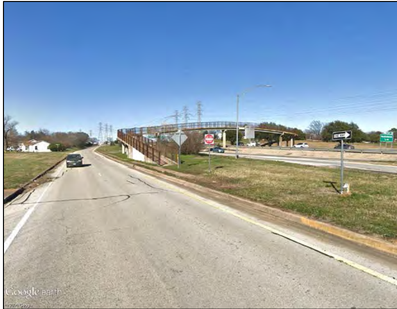
Photo ID 15: View of bike/pedestrian bridge and lack of protected crossing across southbound I-820 frontage road looking north.
